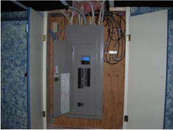
6.0 Picture 1 View of the main electrical panel.
