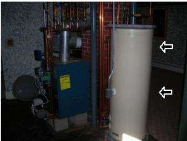
4.0 Picture 3 Combined hot water storage tank from boiler.
