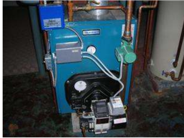
4.0 Picture 2 Burnham oil fired boiler with a Beckett oil burner.
