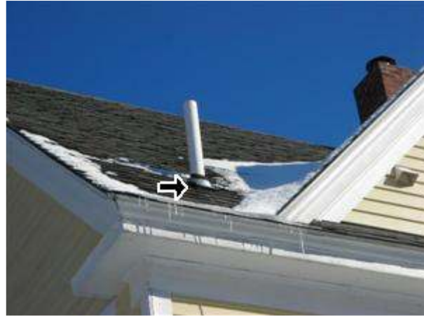
1.0 Picture 4 Bottom of vent stack flashing needs better attachment to shingles
