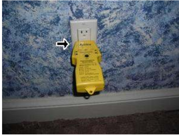
6.0 Picture 2 (5) outlets not grounded.
