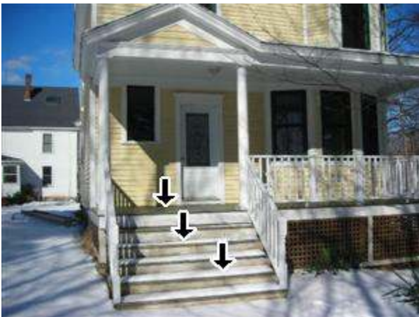
2.0 Picture 5 Front steps and decking need to be scraped and painted.
