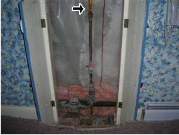
5.0 Picture 1 Main shut off valve for the water supply, located in the basement.
