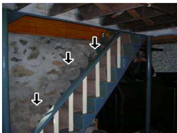
3.0 Picture 1 Better safety railing for basement stairs should be installed.
