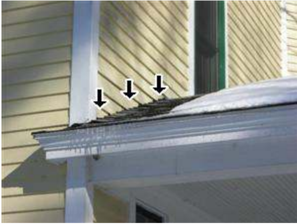
1.0 Picture 3 Step flashing missing, left of front porch, may require repair.
