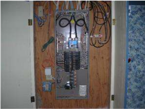
6.0 Picture 3 Interior view of the electrical panel.
