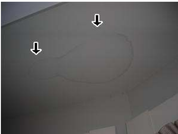
7.0 Picture 3 Past evidence of water penetration near bay window.
